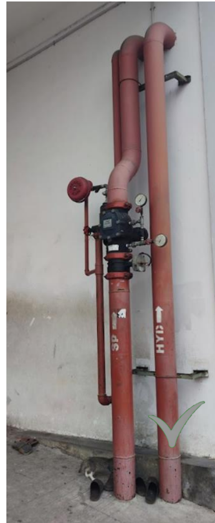
Tersedia pipa sistem hydrant ( fire hydrant ) dan pipa sistem sprinkler
